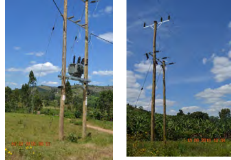
Power transformer and power line in Eastern Ward
